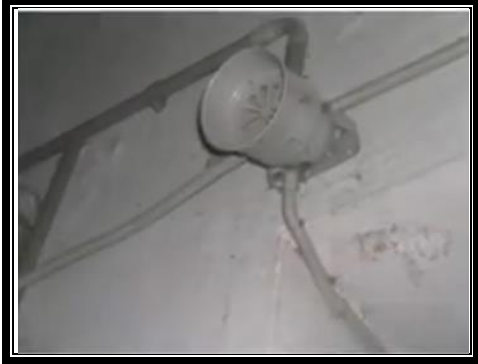
Fig.8. Fire alarm system
